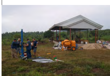
Work on Balut Island is shown here in this photo. In the foreground is the water well drilling rig with the men working. The building is in the background with ongoing work inside on the floor.
