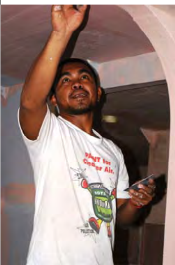
One of the men, a real craftsman with finishing, is applying the 'masilia' (body filler) that makes the walls so beautiful! After sanding this will be painted white.
