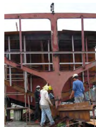
Continued work on the new missionary sailing ship shows workmen setting one of the rib frames in the aft section of the vessel.
