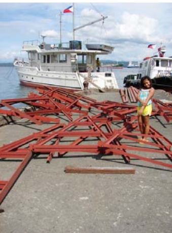
RIM Nativa and Juli at Sta. Ana Pier, February 6, 2012...loading building framework for the church on Balut Island at Port Maveas.
